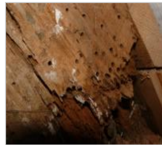
Death watch damage to roof beam
